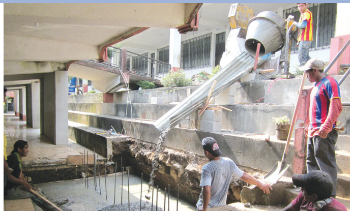
Local workers building a wall for the Carroll EWB earthquake reinforcing project at La Asuncion School in Guatemala. A goal of EWB is to train the locals to work on the project themselves.
