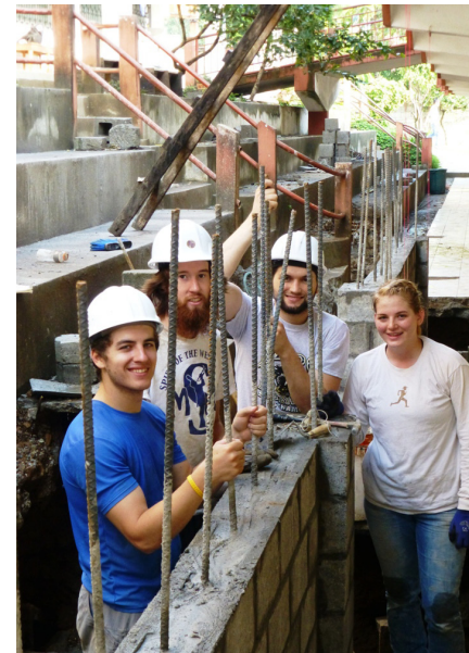
Above: On the fourth construction day, a wall reaches 4-feet high, marked by (left to right) Carroll EWB student Evan Tremaine, alumnus Jennings Anderson, and students Brian Murphy and Whitney Miller
