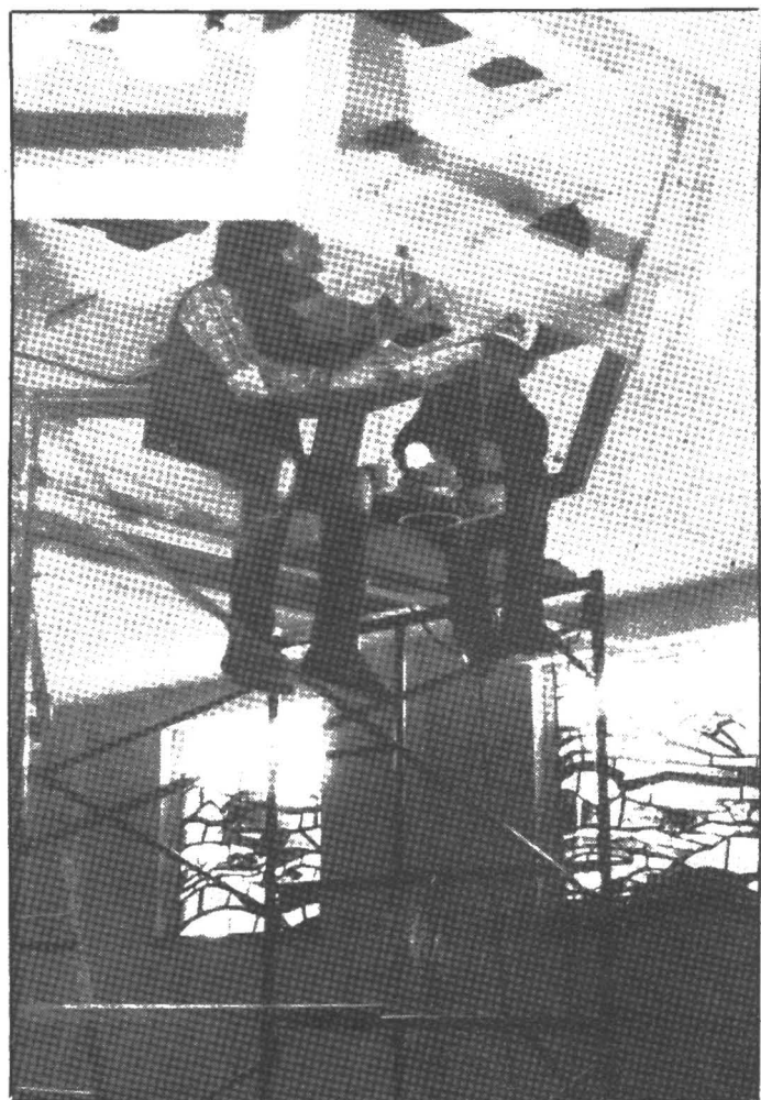
Two men, while working on the new Guadalupe Chapel, were blown into the ceiling. Later, scaffolding was erected around them to make their situation less uncomfortable, until emergency aid arrived. photo by Bridget Moylan
