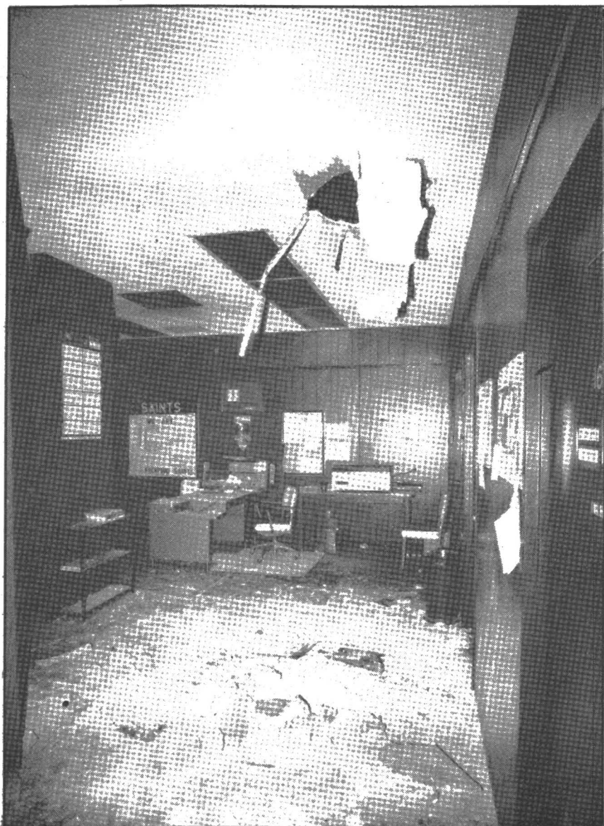
Debris penetrated even the office area of the P.E. Center. Photo by Bill Sallaz.
