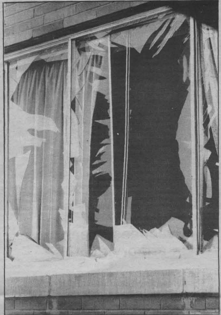
Shards of glass frame a Guad window. (Photo by Bill Sallaz)
